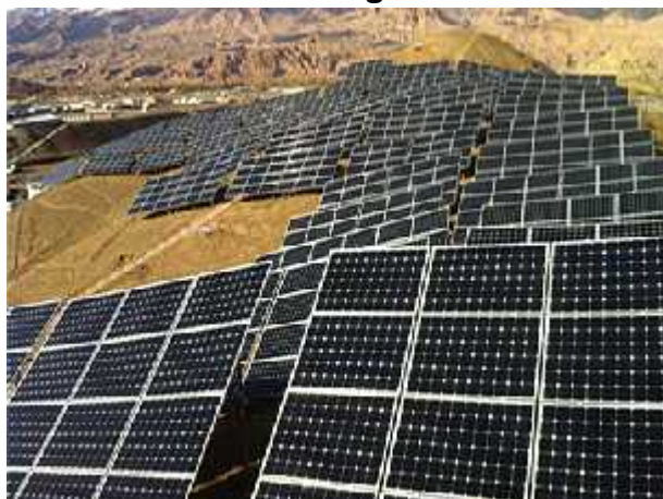
1 MW Installation in Bamyan Province in Central Afghanistan
